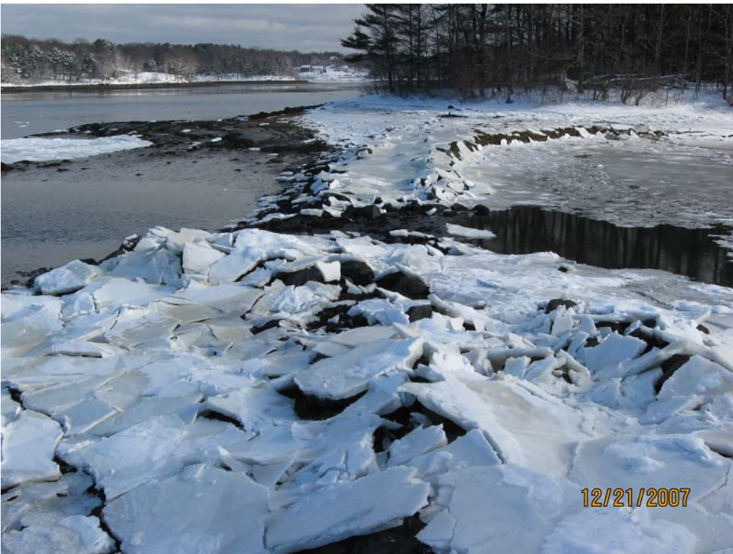
Dam on ebbing tide showing breach.
